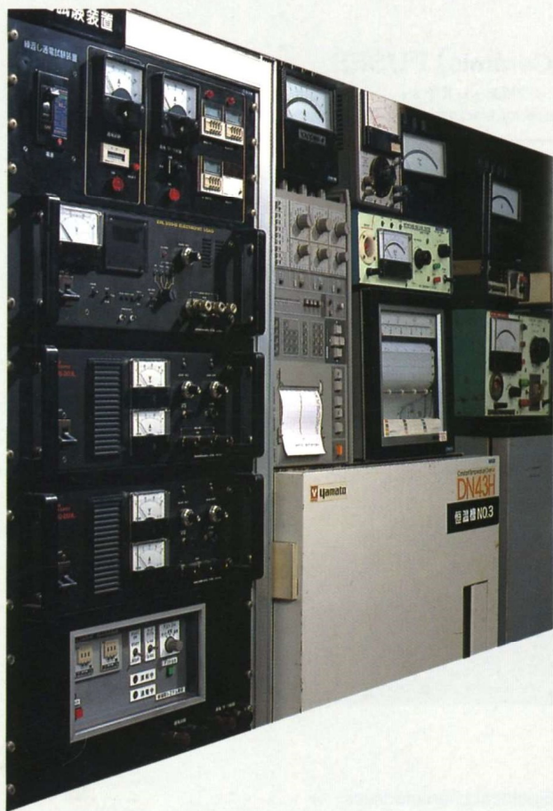
通電試験設備 Loading test equipment
